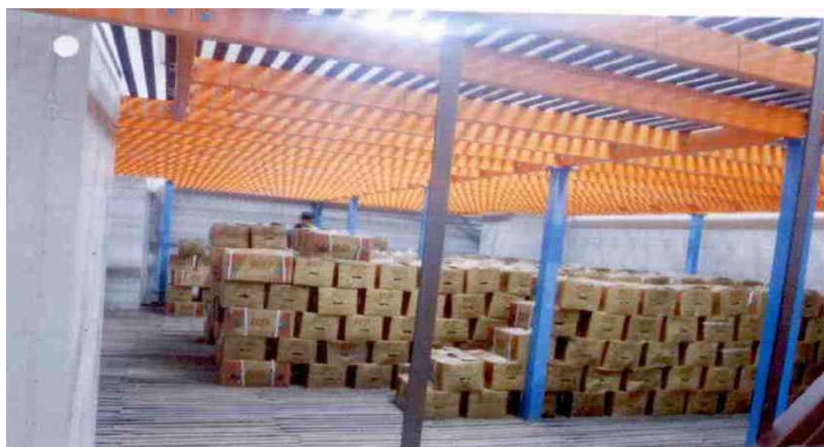
NHB assisted Cold Storage in Jammu & Kashmir
